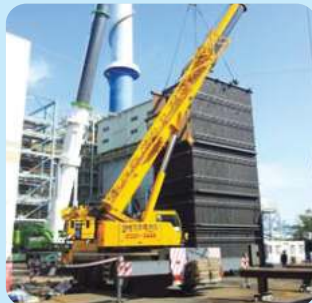
폐열보일러 WASTE HEAT RECOVERY BOILER
