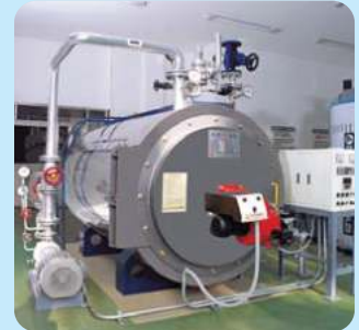
열매체보일러 HOT OIL BOILER
